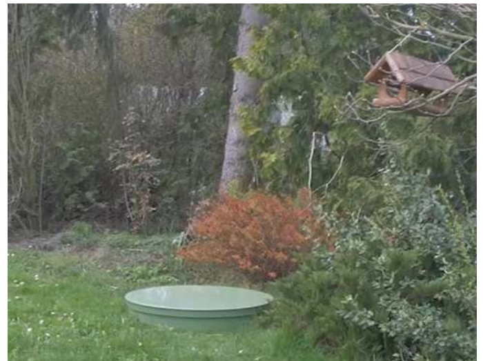
Installed WWTP PRIME 7
